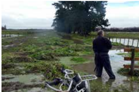
... and then it rained. Blocked Culvert. Paddocks waterlogged. Booked diggers (6 months) were always coming next week. April 2018, OSRS
