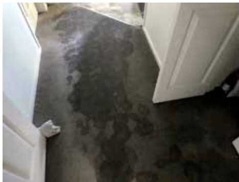
Homestead flood pre-Christmas. Fridge water pipe split and caused hall, carpet and kitchen floods. Industrial blowers huffed for 48hours. No damage.
