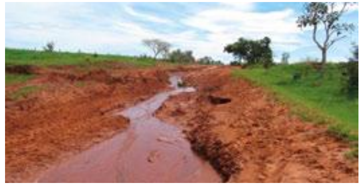
Many secondary roads become rivers regularly. Mato Grosso do Sul
